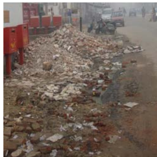
(11) Construction waste On roadside
